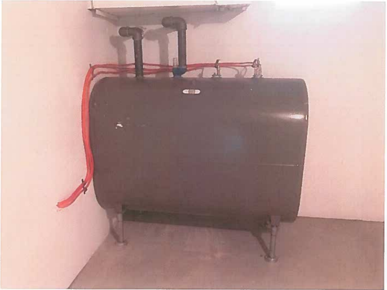
Photograph #5: New Granby 275 10 Year tank installed in basement
